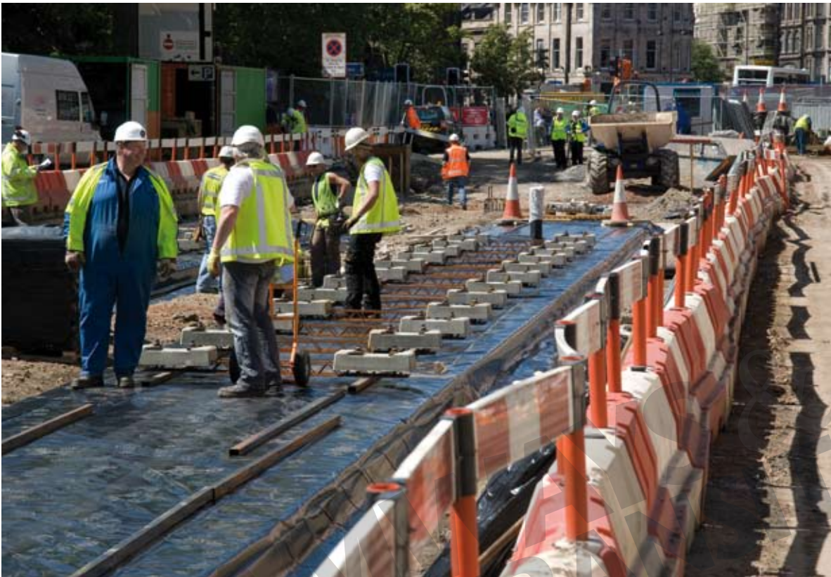
The UK's current major new tramway project: tracklaying takes place in Edinburgh city centre during summer 2009. TIE
