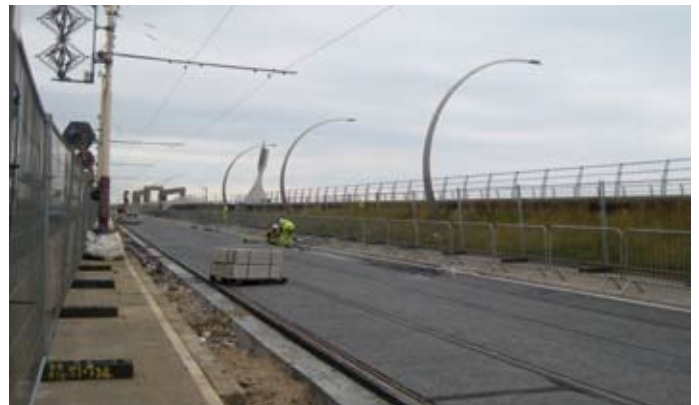
This new track is on the Blackpool Tramway between Pleasure Beach and Starr Gate, with contractors at work on 18 June. The tramway is overlooked by Blackpool's modern artworks in the 'Great Promenade Show'. Barry McLoughlin
