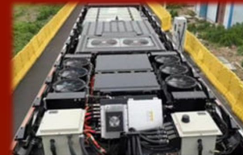
The hybrid power system on the roof
