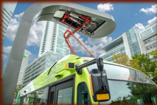
Overhead charger for Tram & Bus
