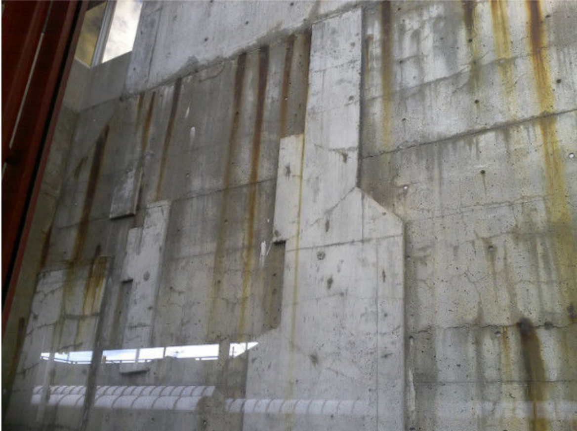
Aging Concrete Retaining Wall at Westboro Station (Photo Credit: Fraser Pollock)
