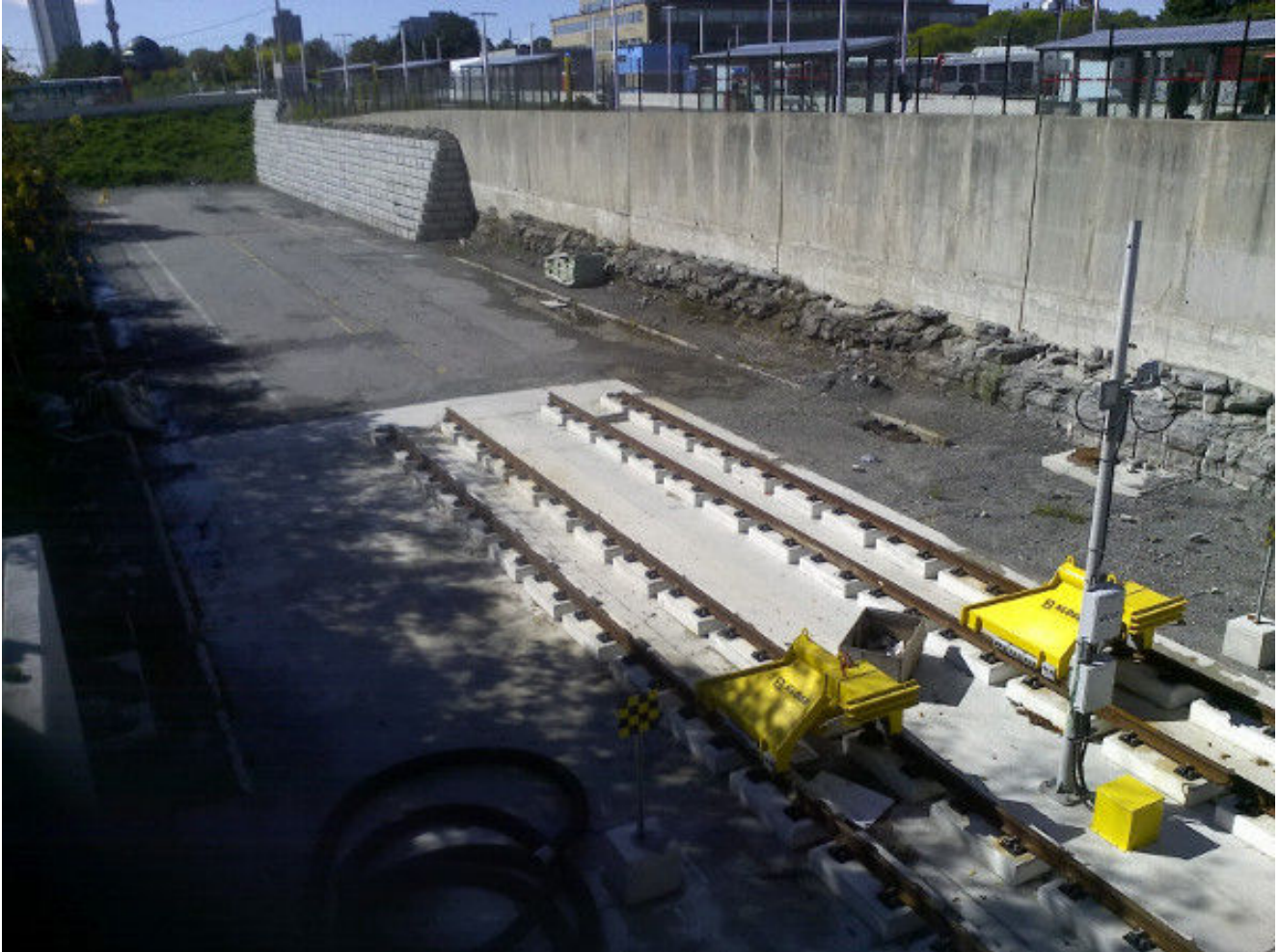
The West end of Tunney's Pasture Station as well as the end of track. Notice how wide the former BRT right of way needed to be compared to the LRT right of way. (Image Credit: Fraser Pollock)
