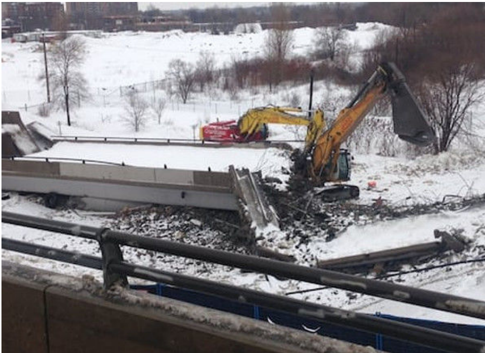
Overpass over Bayview O-Train Station collapsed when it was being dismantled in March 2016 (Photo Credit: CBC Ottawa)
