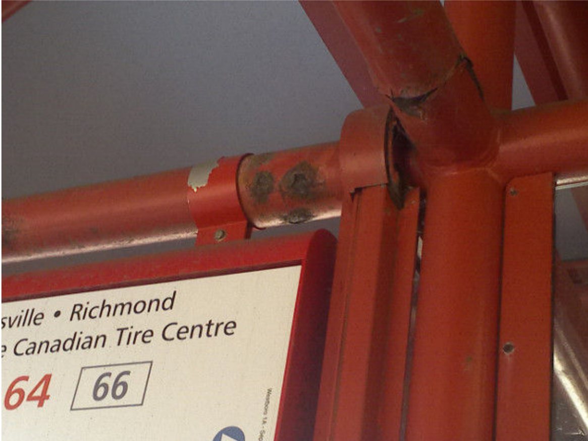
The red steel structural tubes a.k.a. "The Tinker Toy" rusting through at Westboro Station (Photo Credit: Fraser Pollock)
