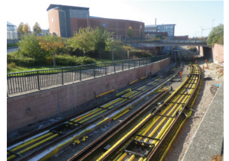
▲ ABOVE: The EMC mitigation system uses feeder cables along the rail, feeding the overhead at each pole.
