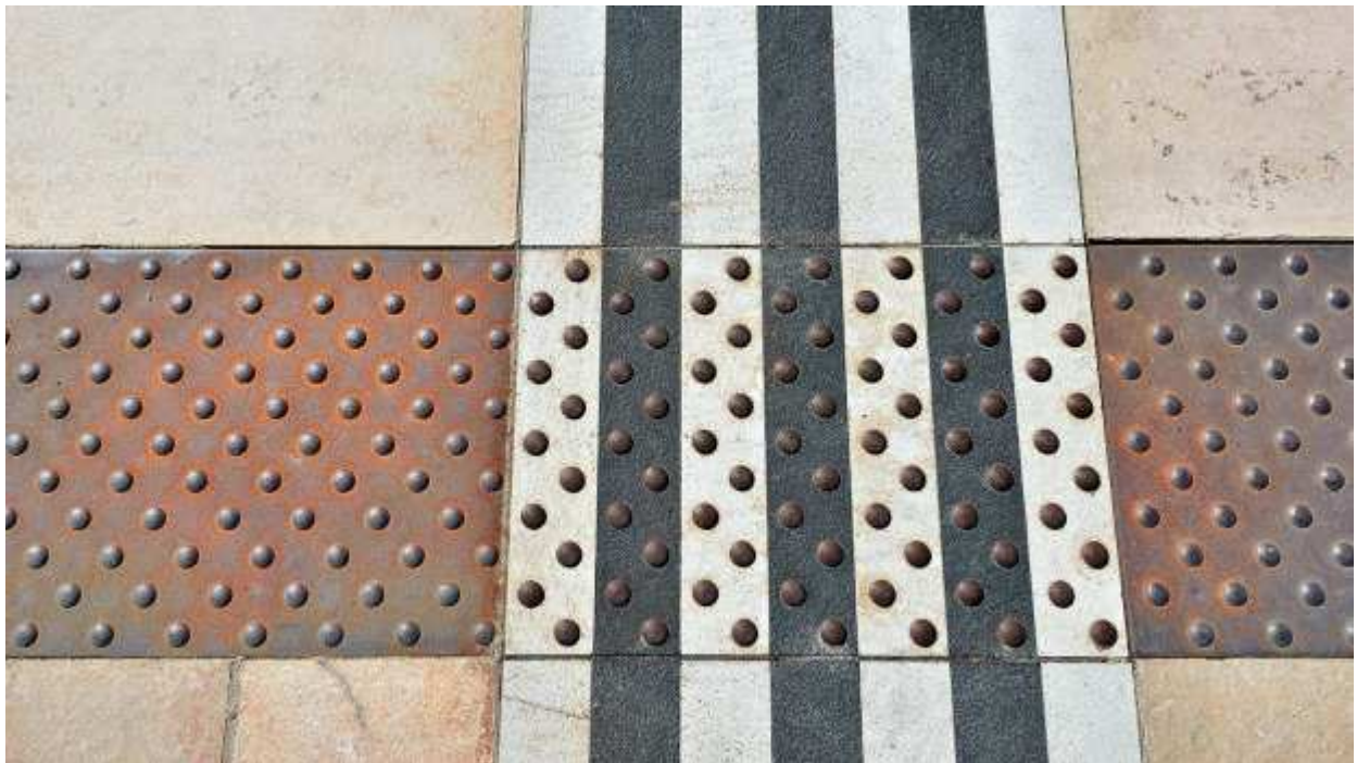
A detail of the paving for the tramway in Tours. Photo: Richez Associes
